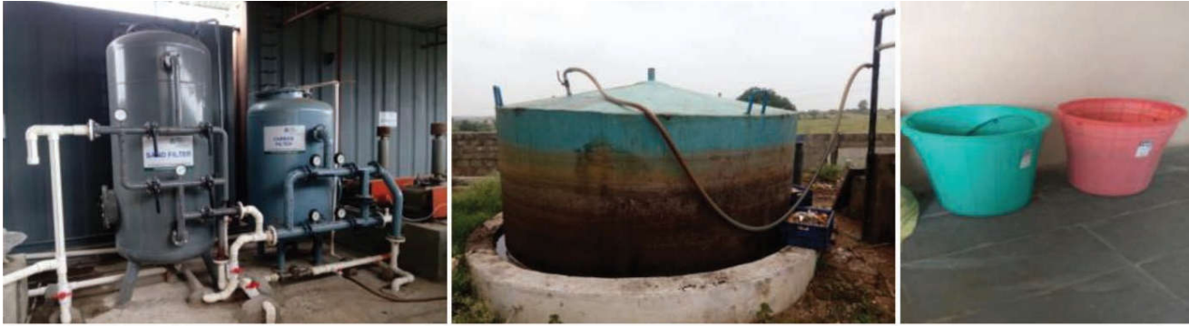
Liquid and Solid waste management plant at GNIT
