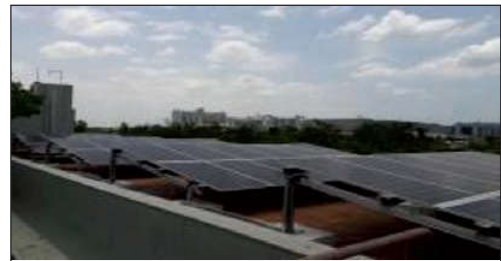
Rooftop solar panels
