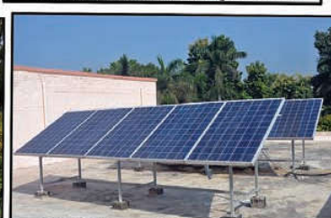
Solar Power Installation on Hostel Roof
