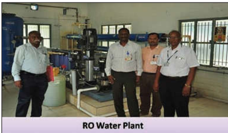
RO Water Plant
